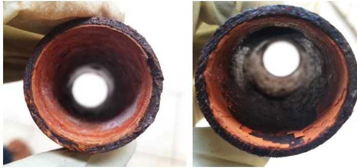
Figure 4a. Scaled tube prior to treatment (left); evidence of scale exfoliation after 2 hrs cleaning (right).
